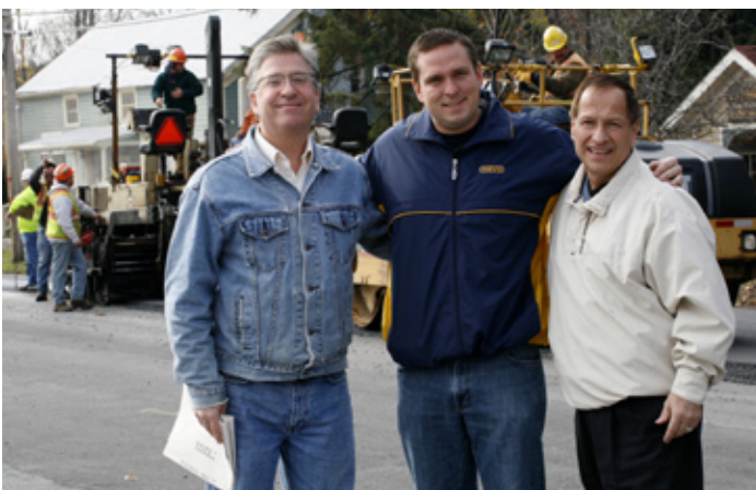
Newly elected Chester Town Board member Matt Kannon, Chester Town Supervisor Steve Neuhaus and Orange County Executive Ed Diana stop by to watch as workers pave Kings Highway in Sugar Loaf.
